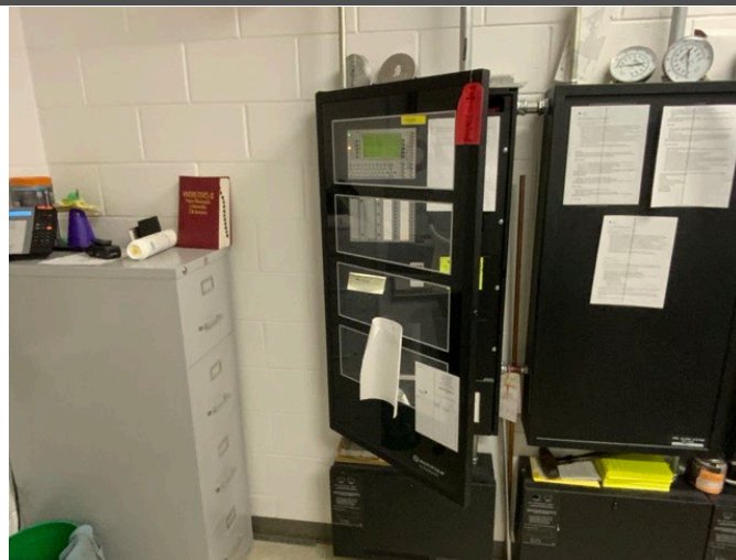
26 - FIRE ALARM PANEL
